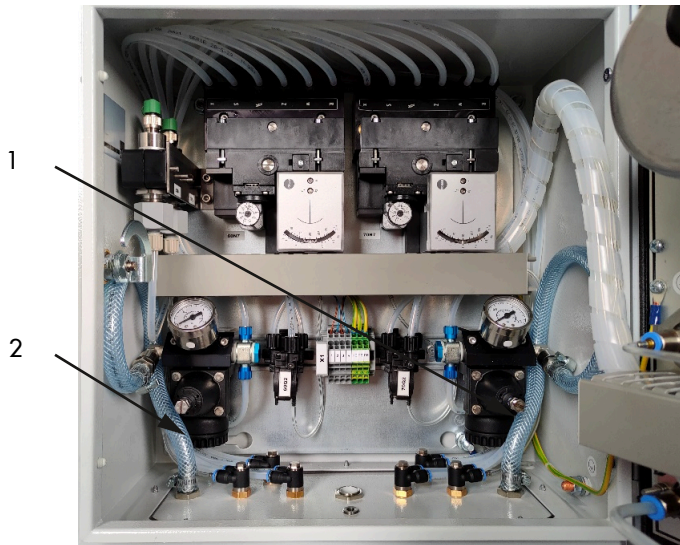
Fig. 15: Setup inside the Type 7311 Air Control System
